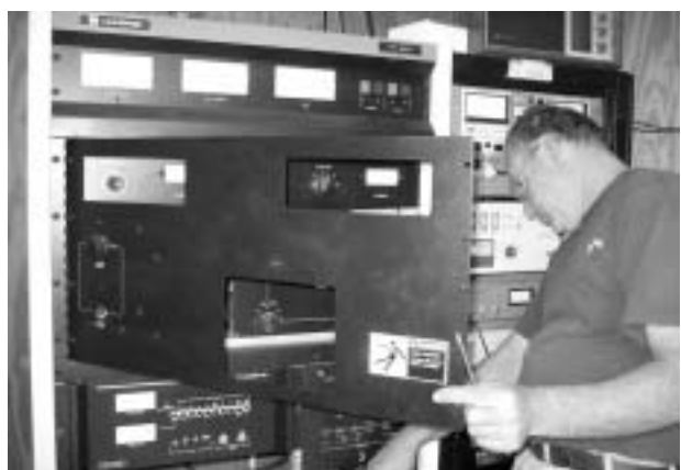
WJFF's engineer, Earle Nietzel, troubleshoots the transmitter on August 14th, following the largest blackout in U.S. history. While WJFF's studios are powered by Jeffersonville Hydroelectric, the tower is located in Liberty and, unfortunately, is on the grid. Power surges and fluctuations took a toll on the transmitter and left WJFF broadcasting at low-power for a couple of days.
